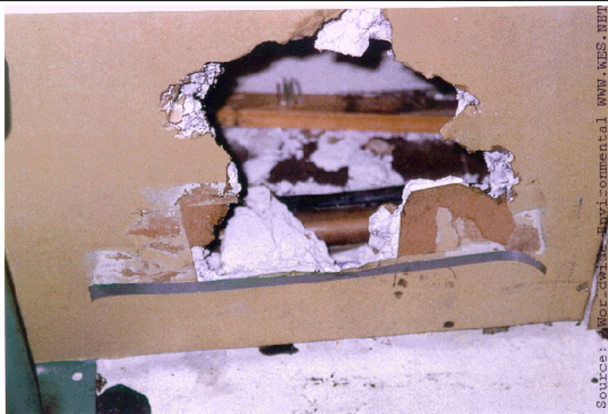
FIGURE 4-3 Dirty Unsealed Subfloor
